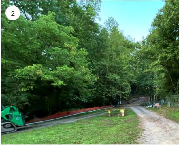
Conduit for new electrical service to wet wells
