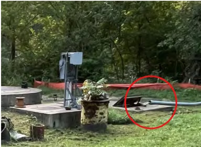
Temporary wiring to raw water pumps
